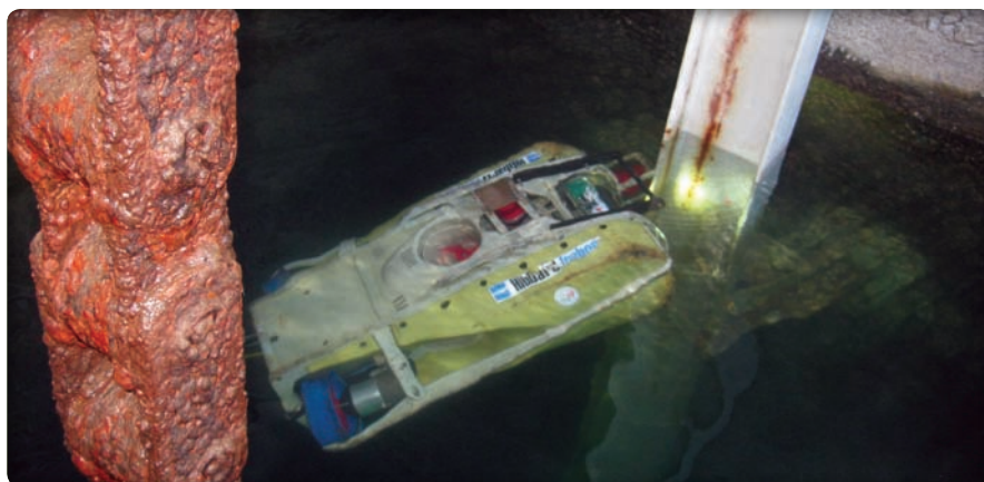
Remotely operated vehicles can be used to perform many tasks at hydroelectric facilities, including inspecting gate valve guides.
